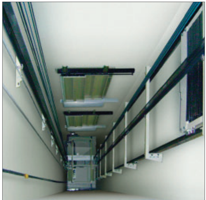
Figure 1: The shaft is a critical area used to control or avoid fire propagation in the building.
