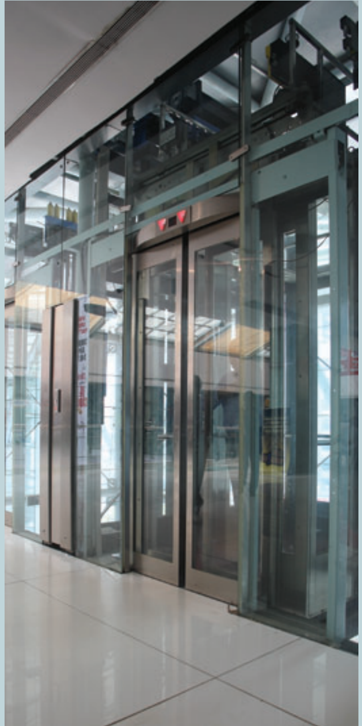
A bank of elevators
